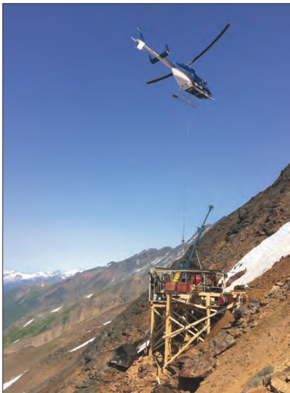
An aerial drop of fuel to a rig targeting the Inel zone at KSP, a gold-silver property in northwestern British Columbia being explored by Colorado Resources Ltd. Encouraged by early performance and results of this drilling, Colorado opted to increase its 2016 program with the goal of earning a 51 percent interest in KSP by the end of the field season.
