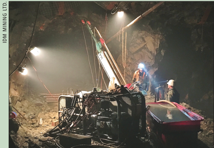
Underground drilling is testing expansion targets adjacent to the reserves at Red Mountain with the goal of extending the life of the mine proposed for this gold project in northwestern BC.
