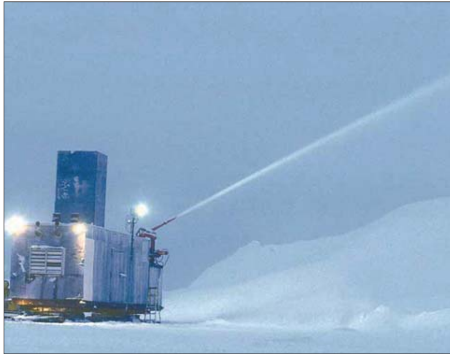
Operators spray water onto the roadway surface to compact snow and build up the thickness of ice roads.
