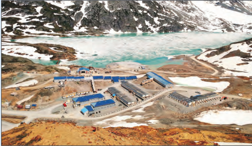
This exploration and development camp at Brucejack is being replaced by a 330-person permanent facility currently being constructed.
