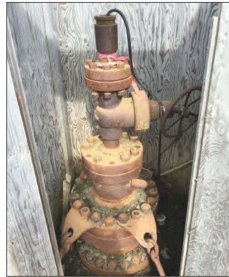
Dilapidated wellhead equipment on the South Barrow No. 2 well, one of the National Petroleum Reserve-Alaska legacy wells addressed by the Bureau of Land Management well remediation program.
