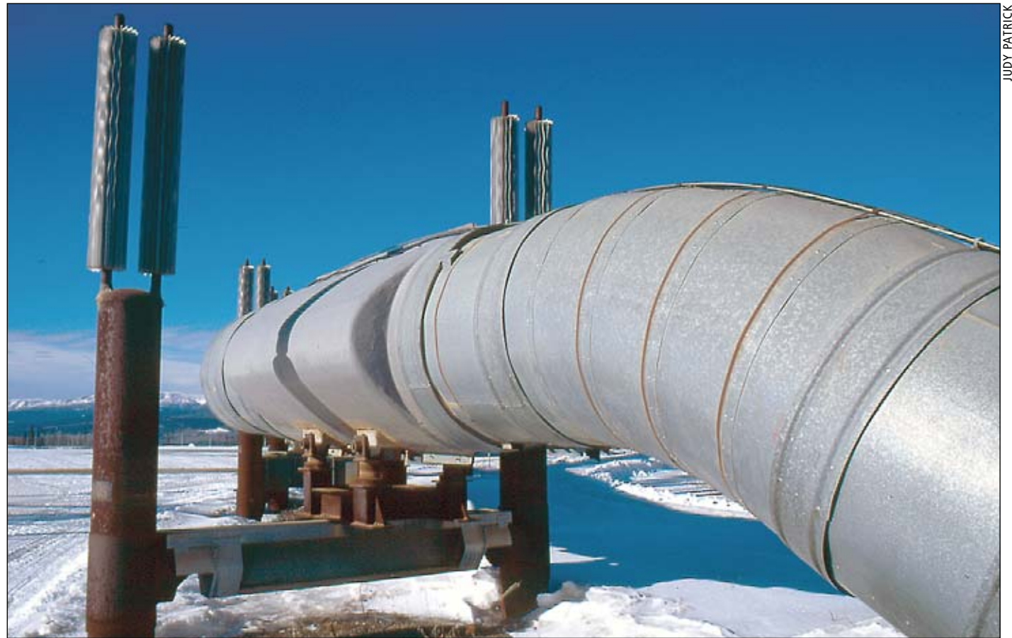
The 800 mile trans-Alaska oil pipeline stretches from Prudhoe Bay in the north to the port of Valdez in southern Alaska.
