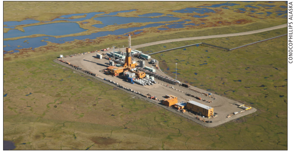
The Doyon Rig 19 on ConocoPhillips' CD3 drill site in the Colville River unit.
