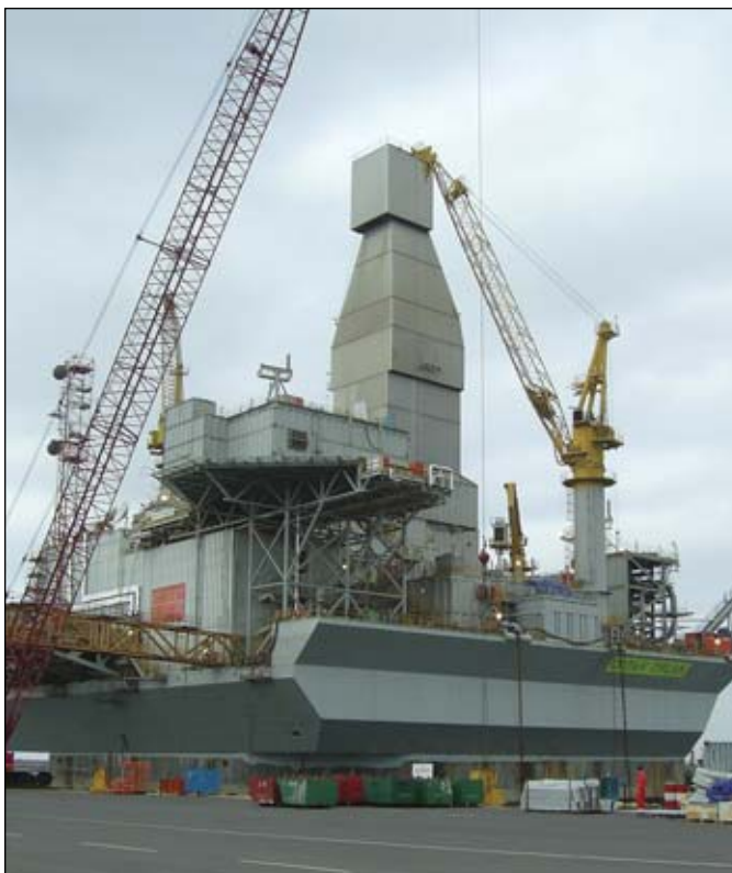
The Orlan Platform at the Hyundai shipyard in Korea. It is a concrete drilling island that had a first life in the Beaufort Sea in Alaska and has now undergone remodeling and upgrading to work offshore of Sakhalin Island. “When I went aboard it in Ulsan, Korea it was like coming home. Many of the crew onboard had worked in Alaska,” Simmons reported.
