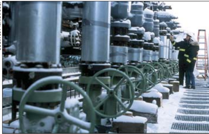
NANA/Colt specializes in providing facility and field engineering and design support in remote locations.
