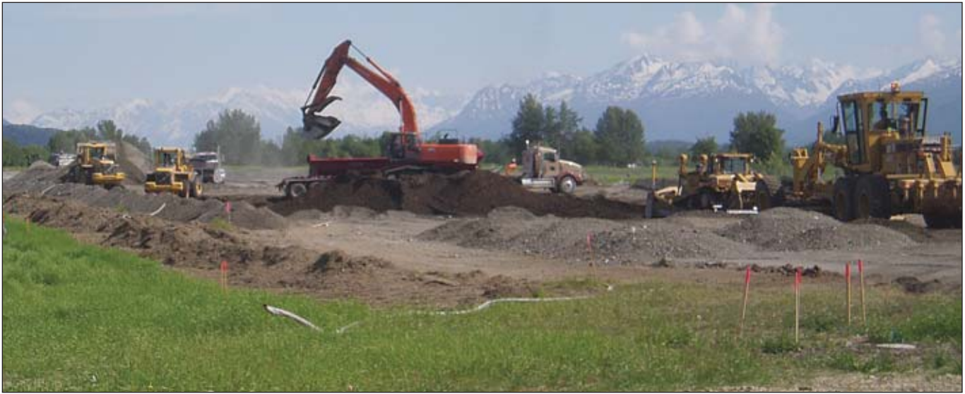
A Cruz Construction crew handles some earth moving at the Palmer Airport
