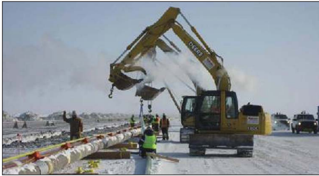
Price Gregory Services Inc. specializes in Arctic engineering and construction like this recent pipeline built to transport crude from the 90 million-barrel Oooguruk unit to connect with the existing pipeline system on the North Slope.
