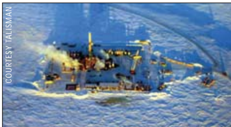
Nabors 14E drilling a successful exploration well in NPR-A during the 2006-07 drilling season for Talisman Energy's Alaska subsidiary, FEX.
