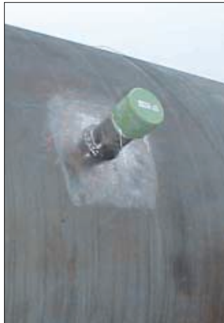
Oct. 7: Permanent repair. A Thread O Ring has been welded onto the pipeline.
