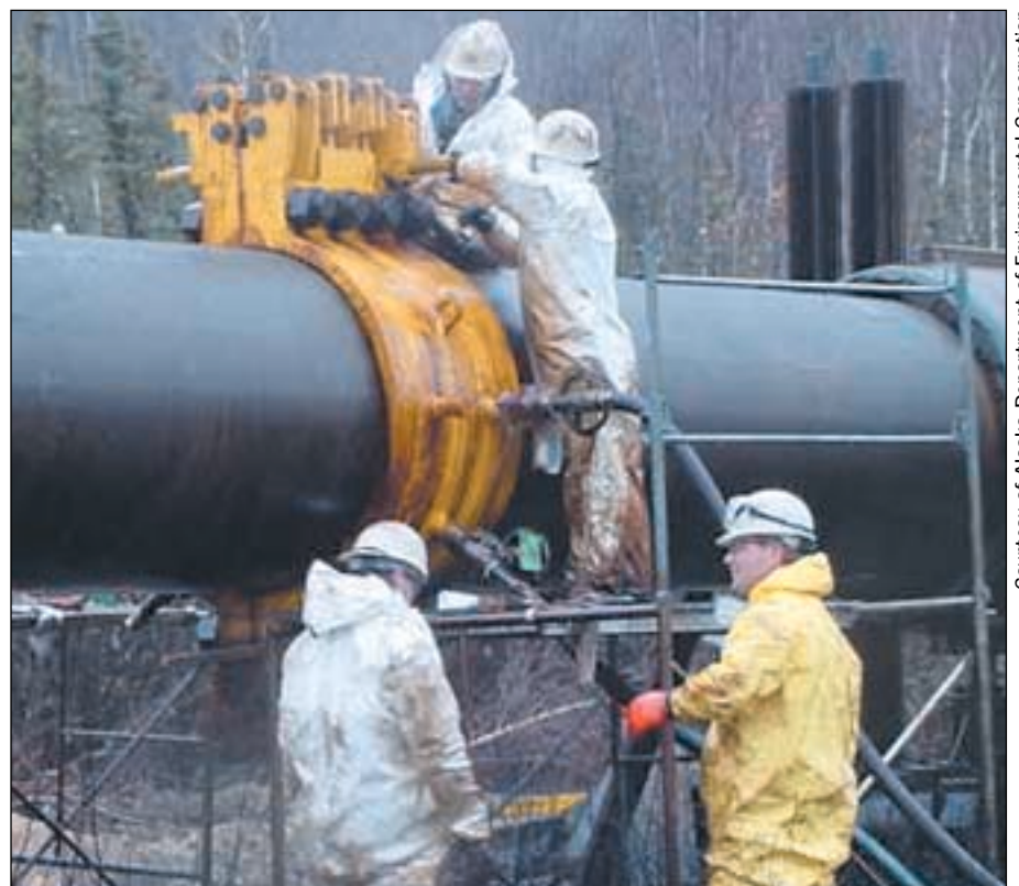
Above, Oct. 6: Alyeska Pipeline Service Co. responders with hydraulic clamp in place on pipeline. Below, Oct. 7: Cleanup.
