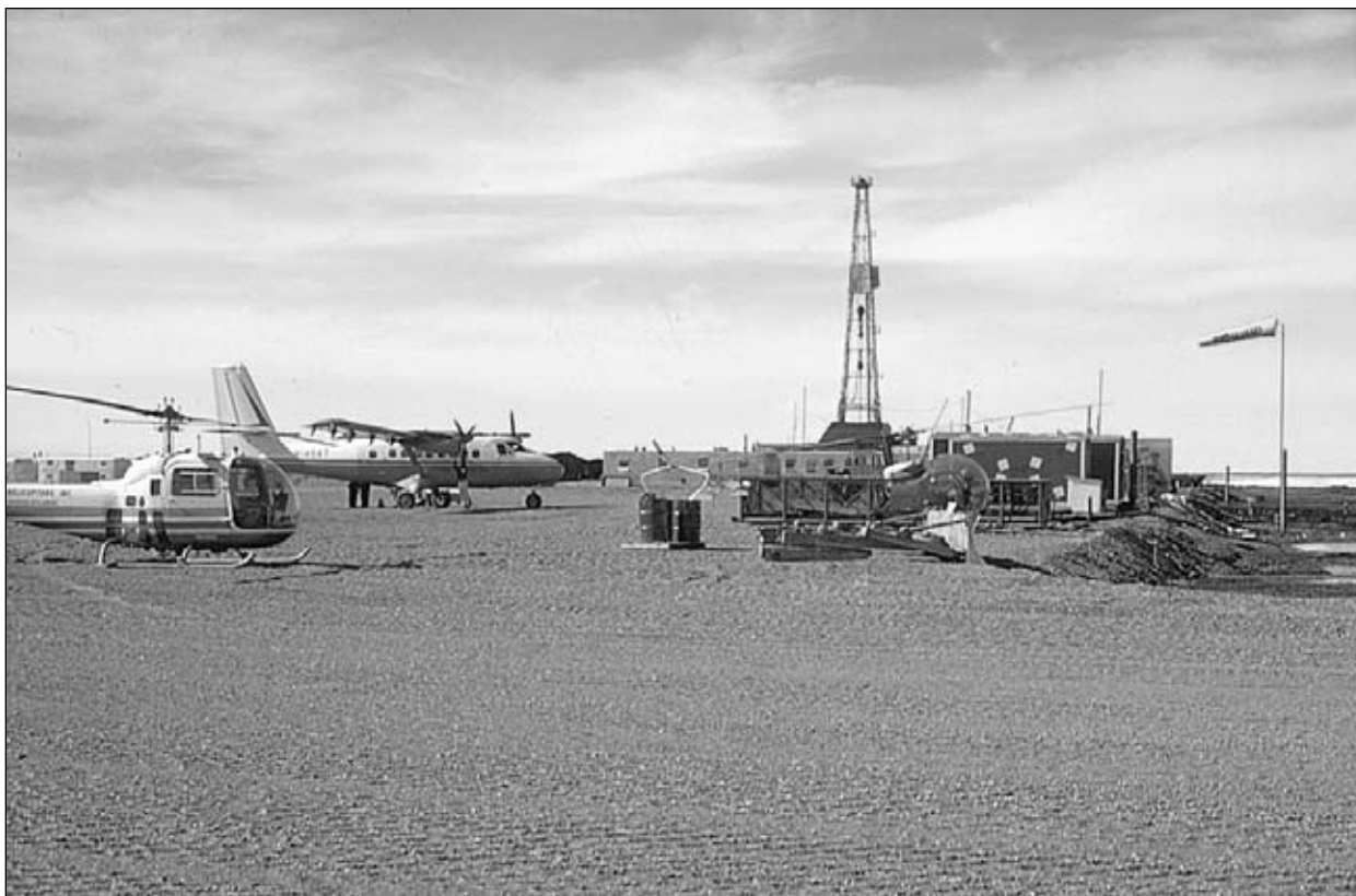
Sag River confirmation well for Prudhoe Bay field, June 1968. The well was drilled by Nabors Rig 9.
