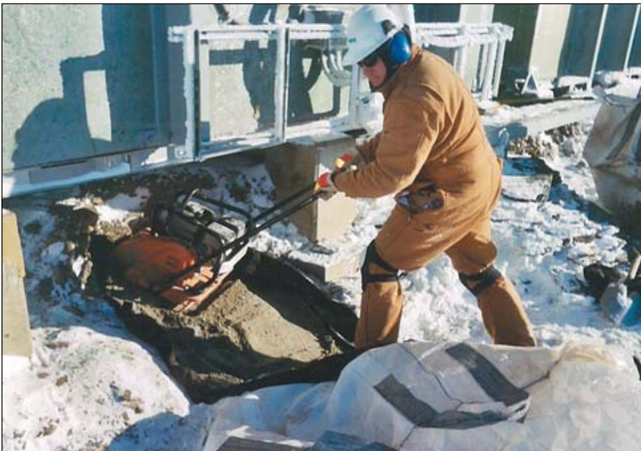
An ENSR worker reconstructs grade at a remedial excavation site after removal of contaminated soil.
