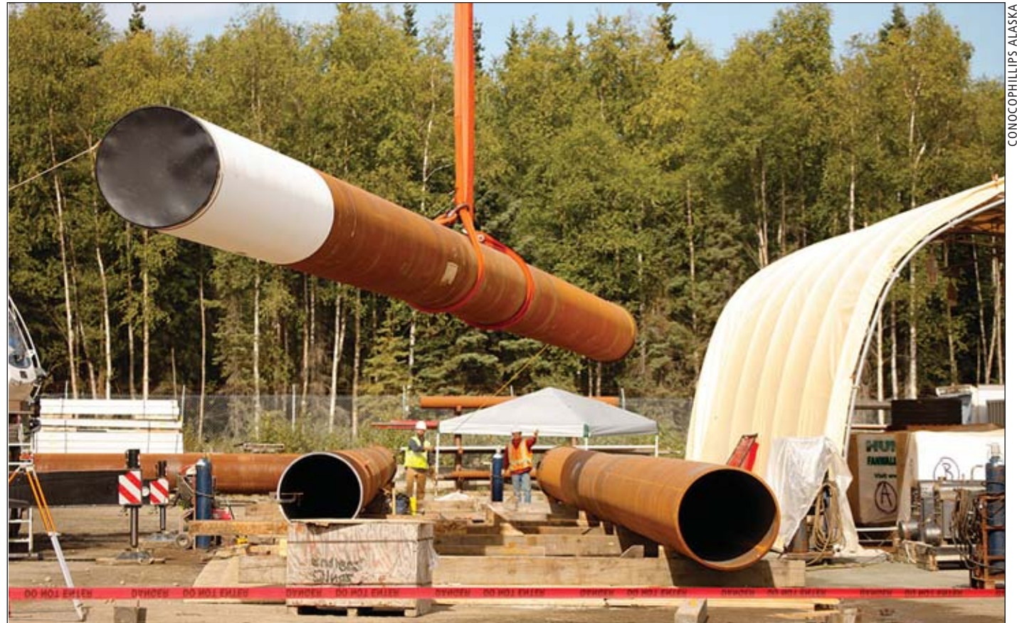
Pipe for pilings for the CD-5 Nigliq Channel bridge staged in Anchorage over the summer.
