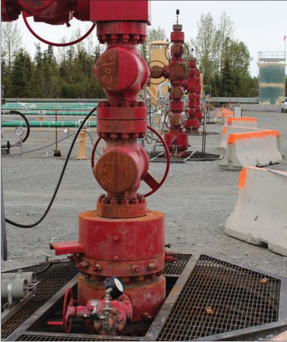
Wellheads in the Cook Inlet Natural Gas Storage Alaska facility on the Kenai Peninsula. The facility's reservoir was filled with gas for use in the winter and has already starting bolstering utility gas deliveries.
