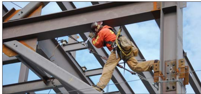
A member of the Pacific Northwest Council of Ironworkers balances carefully on a girder while working on a steel structure in the Seattle area. The ironworkers and the companies that employ them have joined forces to market their expertise.
