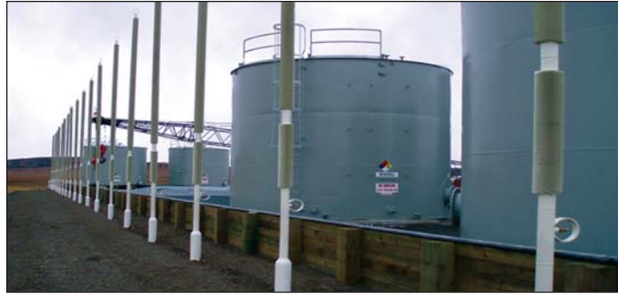
Arctic Foundations Inc. installed these 19x 200SF radiators in a Flat-Loop Thermoprobe system during an upgrade of a bulk fuel facility in Unalakleet.
