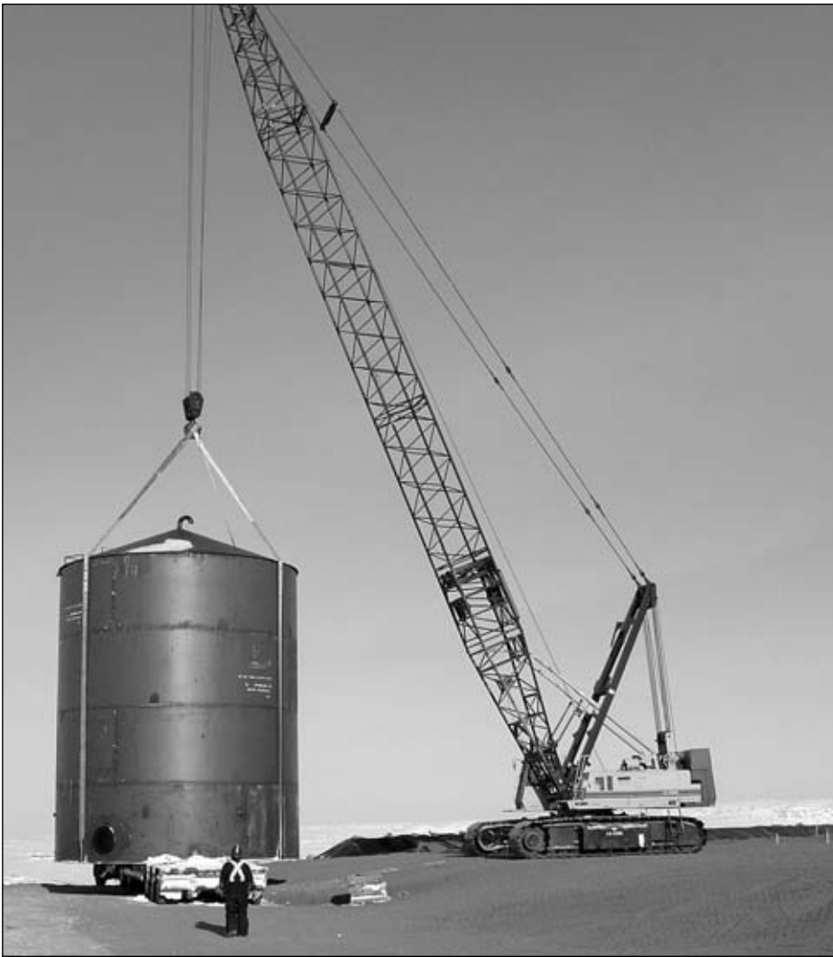
Tahera Diamond Corp. moved 550 truck-trailer loads of goods, including this fuel tank, to the Canadian Arctic for the Jericho Diamond Project.
