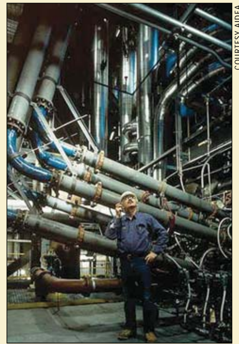
The Healy plant was constructed in 1997 after winning a U.S. Department of Energy grant for clean coal technology projects. It was designed to produce up to 50 MW of power
