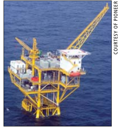
The Falcon Nest platform is owned and operated by GulfTerra Energy Partners.
