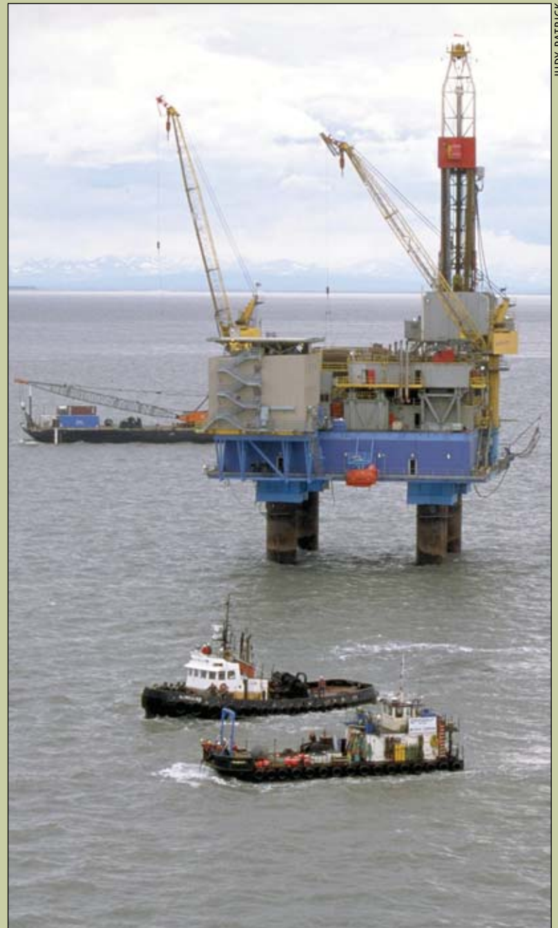
The Osprey platform during the pipeline installation phase. Crowley Alaska's tugboat, Sea Breeze, and American Marine Corporation's vessel, Shamrock, both were instrumental in the pipe pulling operation.
