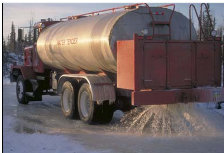
Palmer-based Cruz Construction building Interior Alaska ice roads last winter. Teck-Pogo hired Cruz to construct and operate a winter ice road this winter that follows the same route up the Goodpaster River valley used by Pogo prospectors during the winter season of 1997-1998.
