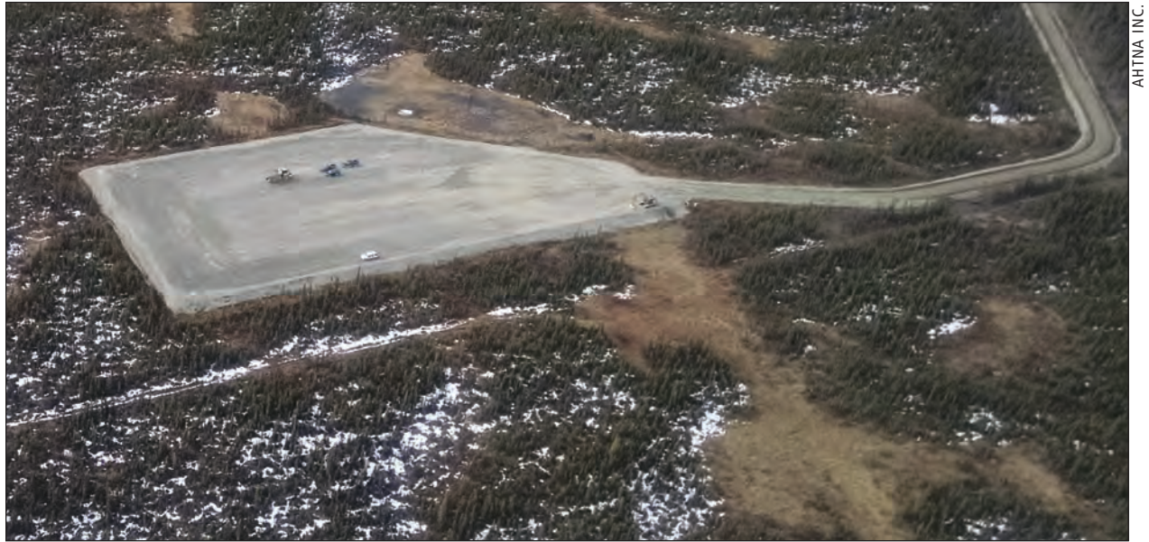
An aerial view of the gravel pad and access road for Ahtna Inc.'s Tolsona No. 1 well, on the north side of the Glenn Highway, 11.5 miles west of the town of Glennallen
