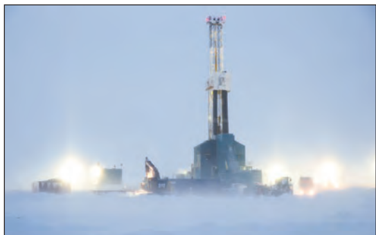
Kuukpik Rig. No. 5 drilling at ASRC Exploration LLC's Placer No. 3 well last winter
