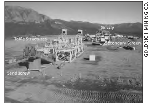
The placer gold recovery plant at Chandalar is expected to process 600 cubic yards of gravel per hour, which will be realized as gravel screens and gold recovery tables are added in stages through 2016.
