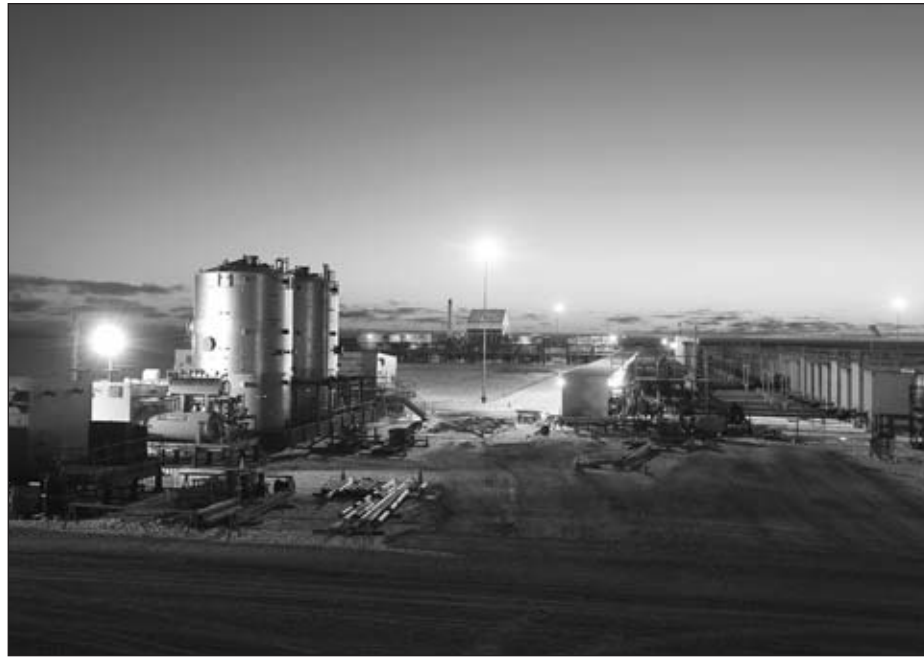
BP's heavy oil test production facility at the Milne Point 5 Pad.
