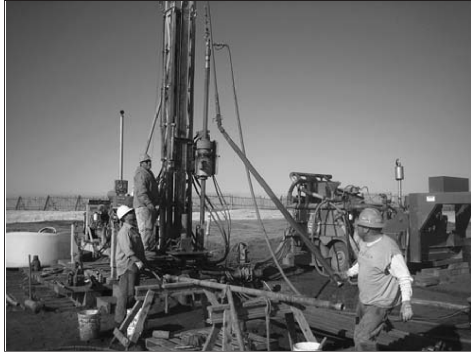
Removing the core barrel inner tube from the Wainwright coalbed methane test well
