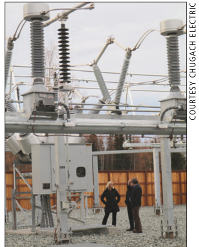
Chugach board chair Janet Reiser touring the substation with Chugach employees Paul Risse and Brian Hickey.
