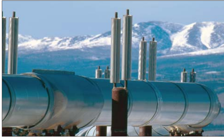
Trans-Alaska oil pipeline
