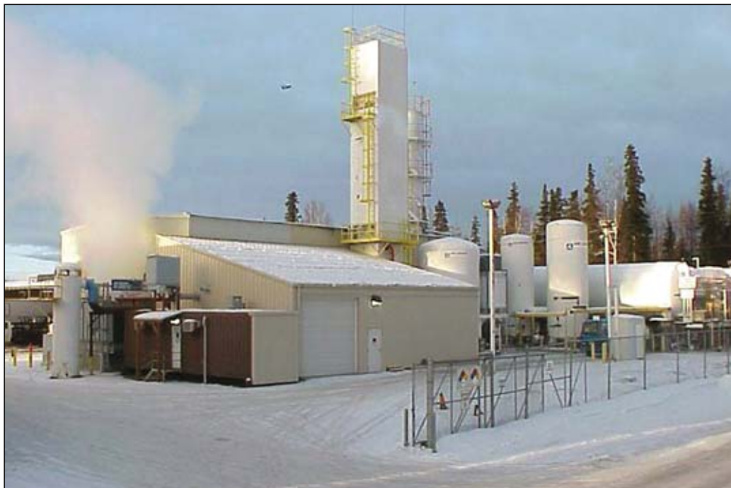
Air Liquide gas manufacturing plant in Anchorage, Alaska
