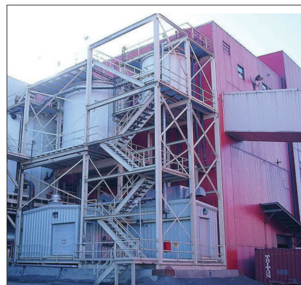
Red Dog's third water treatment plant is reducing total dissolved solids in the mine wastewater.
