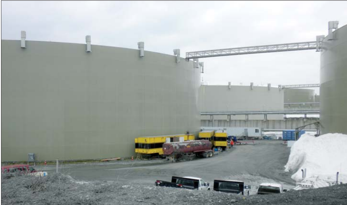
Enormous oil storage tanks at the Valdez Marine Terminal hold North Slope crude until it can be loaded onto tankers for delivery to refineries. Each tank has a capacity of 510,000 barrels.
