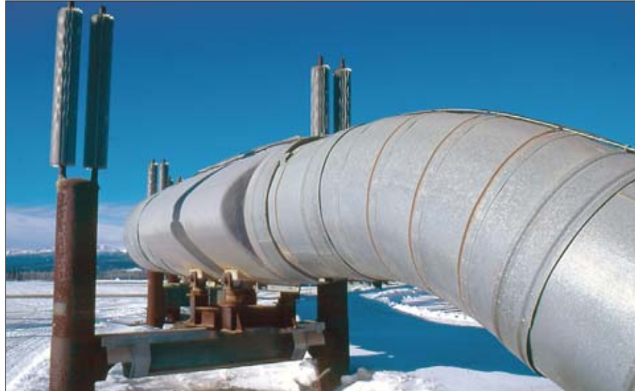
The trans-Alaska oil pipeline
