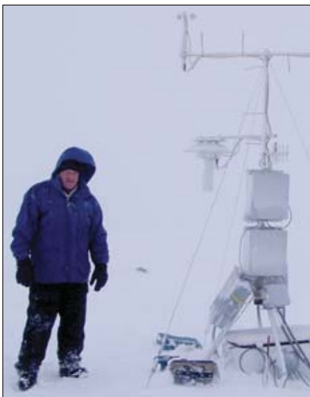
Eric Brudie, a lifelong Alaskan, is a field engineer with the Hoefler Consulting Group who helped install the weather stations for the Pebble project.
