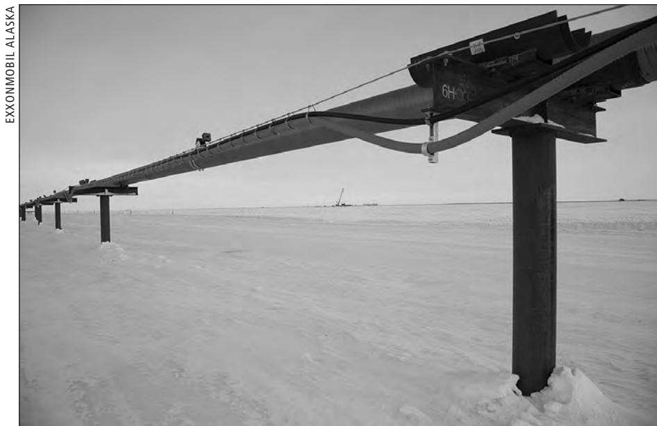
The export pipeline from the Point Thomson field has capacity to handle up to 70,000 barrels per day of condensate, a light form of oil. Initial field production is estimated to be 10,000 barrels per day.
