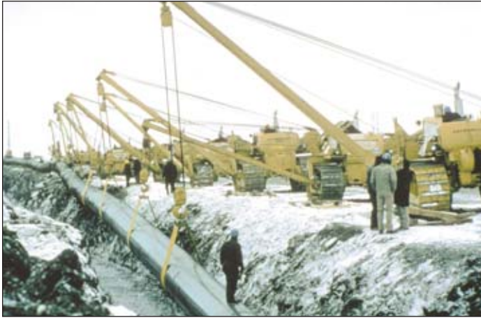
On March 27 the first pipe is laid at Tonsina River. A total of 534 rivers and streams were crossed in the construction of the 800-mile trans-Alaska oil pipeline..
