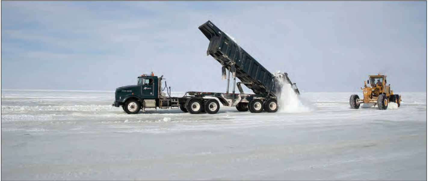
A truck lays ice chips for construction of an ice pad for the Willow project. April 2023.
